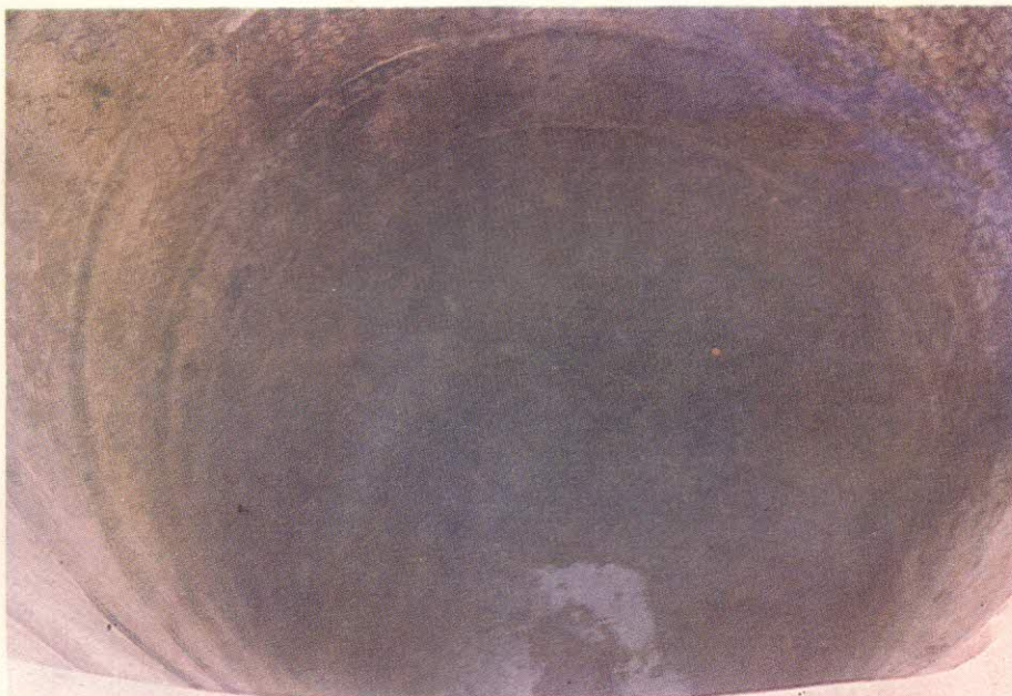
PHOTO 8 : MIS-USED WELL AT PERNAMPET (23030)
