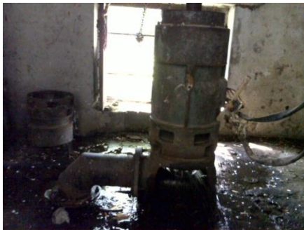
Infiltration well (TR 02) at Pool Side, M A Stadium
