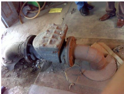
Infiltration well (TR 03) at Company Bagh
