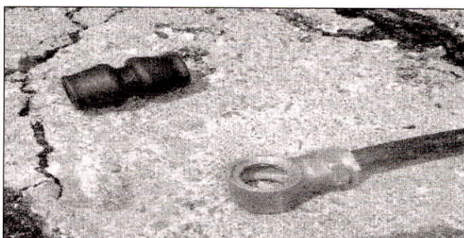
Fig. 2: plastic and brass ferrule sockets where most of leaks occur in house connections
