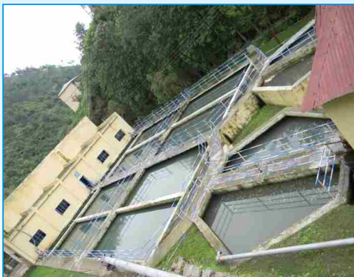
Ashwani Khud Water Treatment Plant (WTP)
