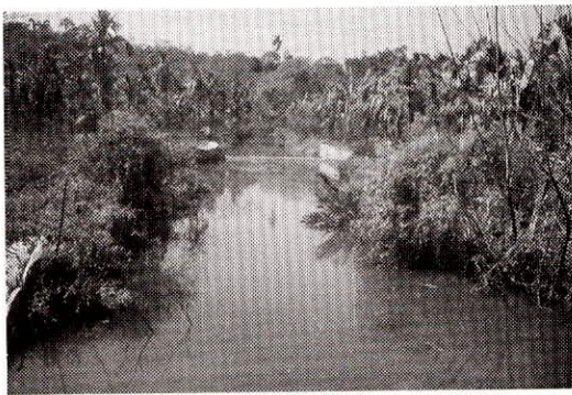
Fig. 16. Check dam affected by tsunami at Chouldari, S. Andaman.
