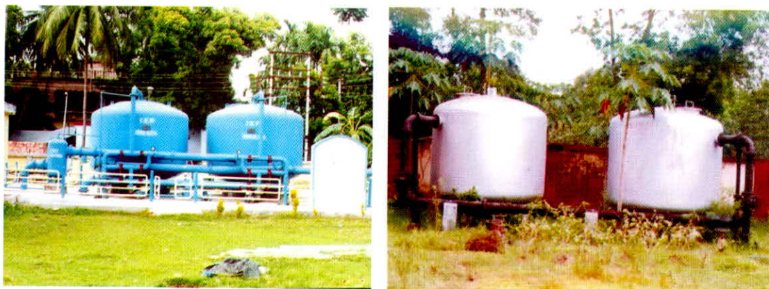
Figure 4.5: Arsenic Removal Plant (ARP) connected to an existing piped water supply schemes (PWSS).
