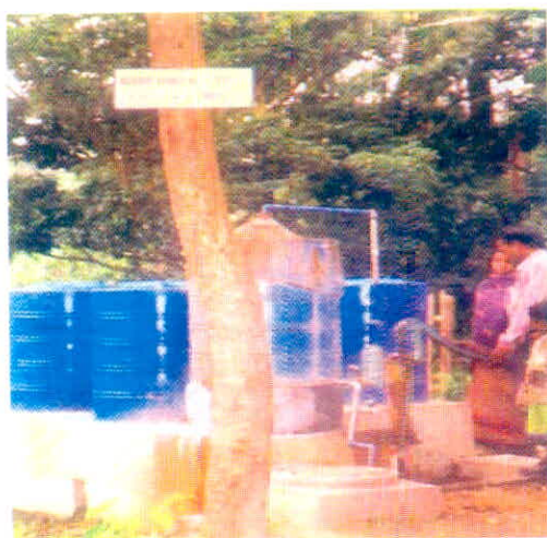
ARSENIC TREATMENT PLANT-PHED MODEL
