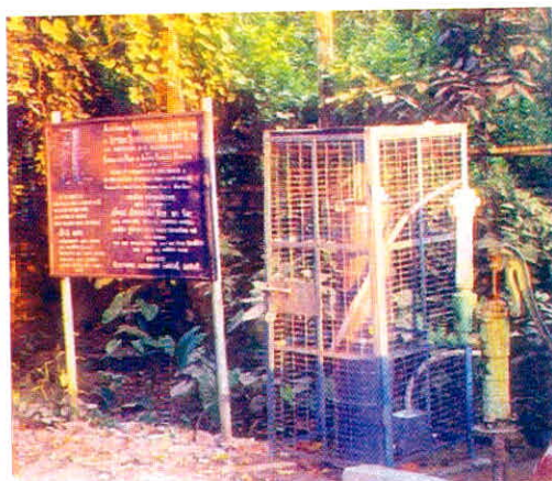
APYRON ARSENIC TREATMENT UNIT
