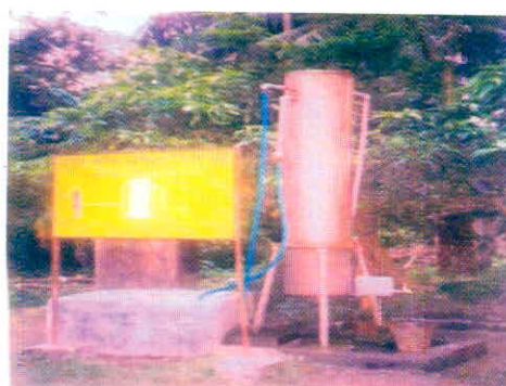
ARSENIC REMOVAL PLANT - OXIDE INDIA
