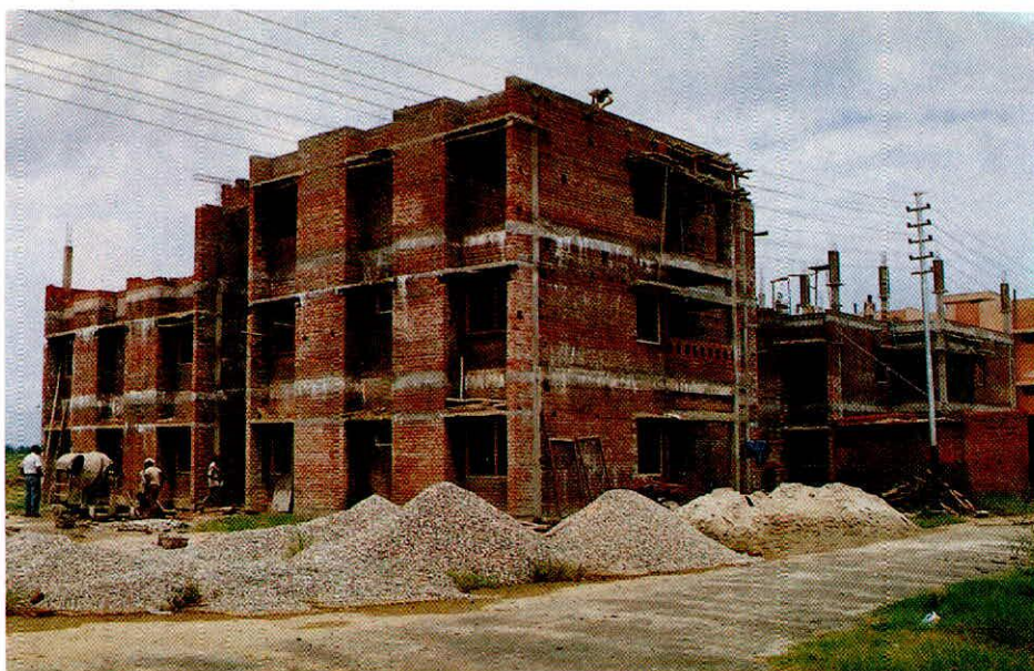
Two Blocks (12 residences) of Scientists' Residences under construction in Institute Staff Colony.
