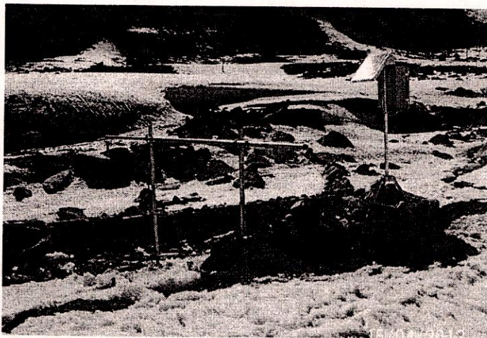
Figure – 2: Radar Water Level system installation by NIH at 4700 m a.s.l. at Ladakh
