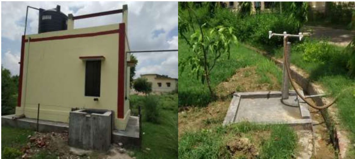
Developed pilot demonstration RBF scheme at Mathura: (a) Pump House, and (b) Stand Post.
