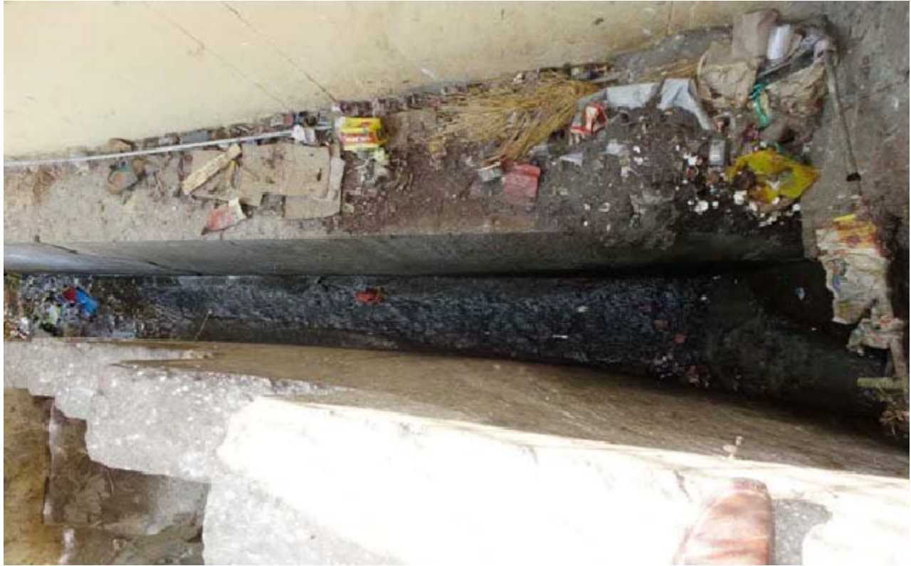
Fig. 8. Open Drain Going in River Alaknanda
