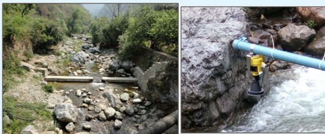
Fig. 2. Construction of compound rectangular weir and installation of AWLR over the Henval stream
