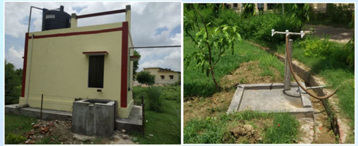
Snapshot of a developed pilot demonstration RBF scheme at Mathura; Pump House and Stand Post.
