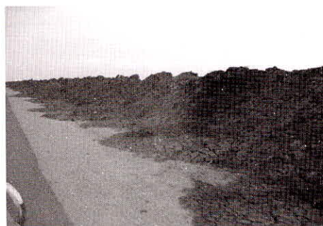
Plate 2: Accumulation of Sediment on Canals Banks
