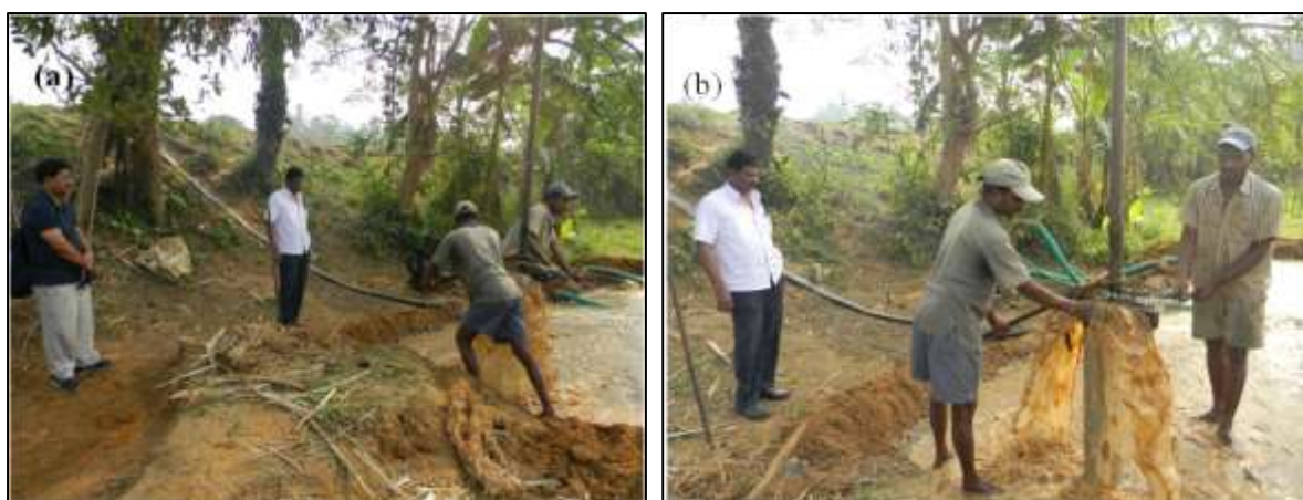
Figure 37: Exploratory drilling of RBF well near Vommavaram village on the left bank of the Varaha river.
