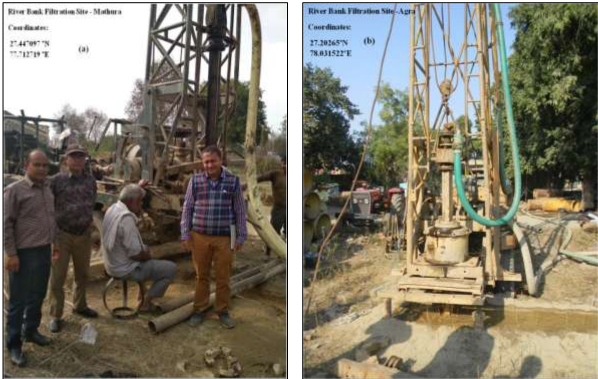
Figure 18: Exploratory drilling by rotary method for RBF well: (a) Mathura (in the premise of UPJNL, near Gakul barrage), and (b) Agra (in the premise of Jal Kal of UPJNL).
