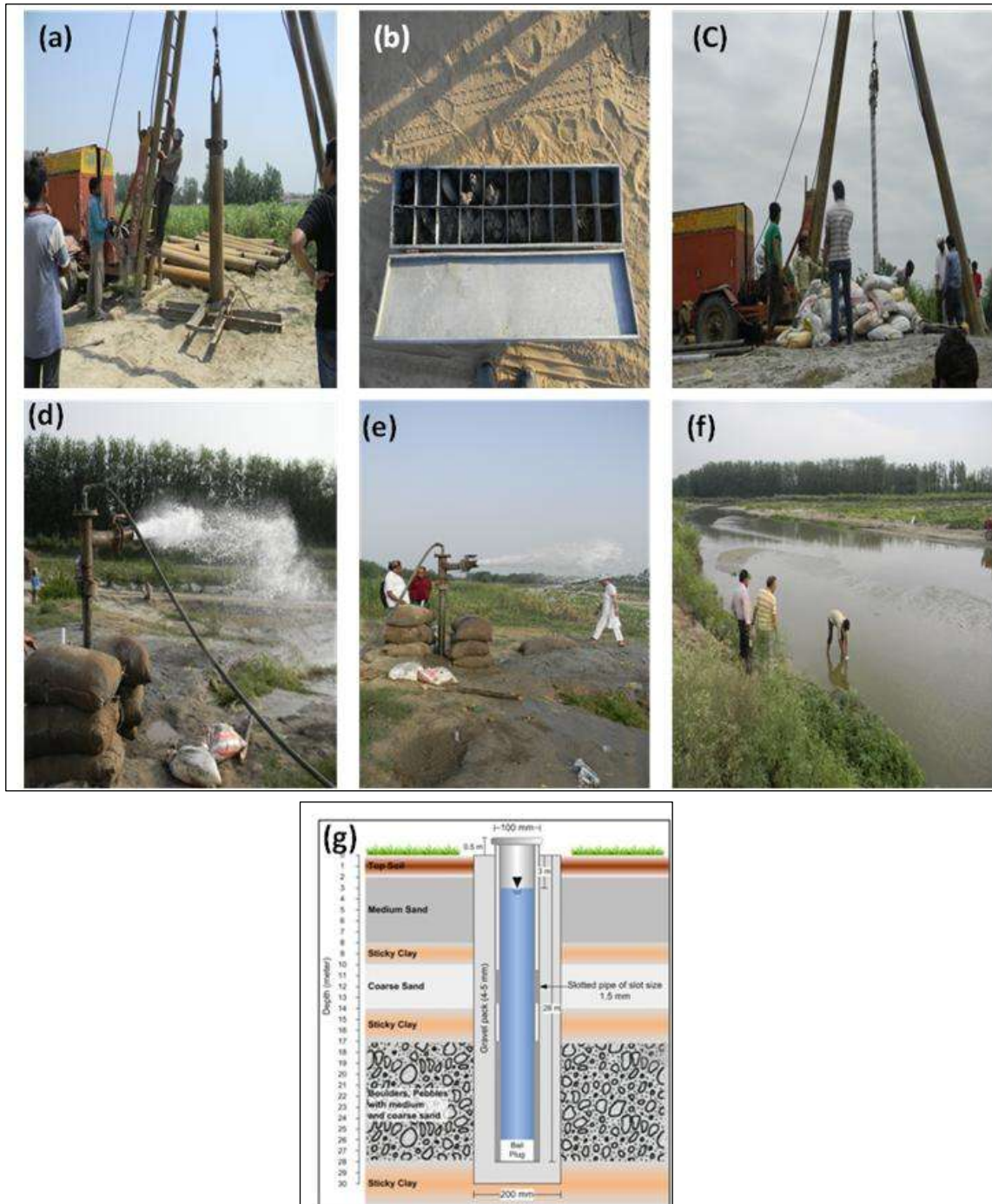
Figure 2 : Few photographs of Kunwa Khera Goan RBF well drilling works: (a) exploratory drilling work in progress, (b) drilled soil cores collected at 1 m depth interval, (c) lowering of tube well pipe in progress,(d) tube well development by air compressor, (e) another view of tube well development by continuous air pressure by compressor, (f) water sample collection from Solani river for water quality detection, and (g) schematic diagram of 20 cm dia bore hole with 10 cm dia lowered tube well and lithological profile of explored geological strata.
