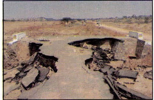
Fig.2. Scouring of soils in flood
