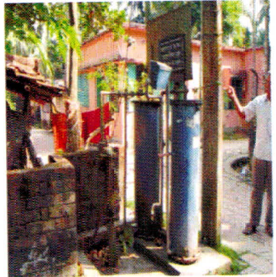
Figure 8.2 : Photograph showing a hand pump connected with similar Arsenic Removal filter located at about one km. distance apart but not under the responsibility of community participation in O & M, found non-functional due to minor maintenance.
