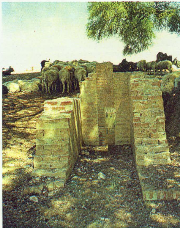
Fig.2 : Exit constructed in the bank of the pond to allow excess water to escape
